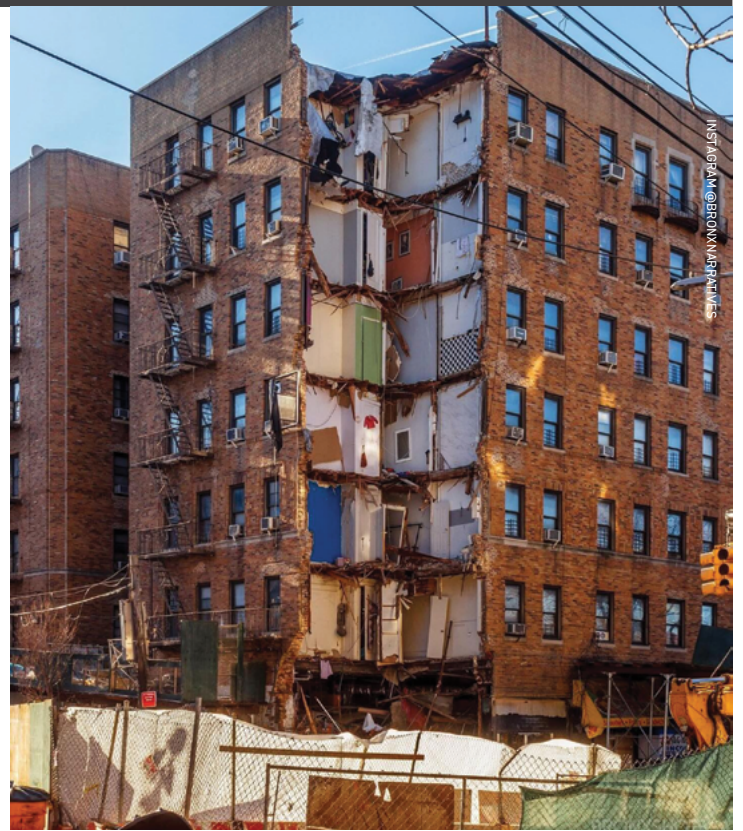
On December 11, 2023, a corner of this seven-story building in the Bronx partially collapsed.
